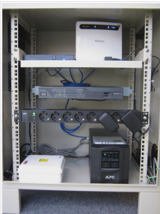
Fig. 2 - Interior de rack AD Rural
