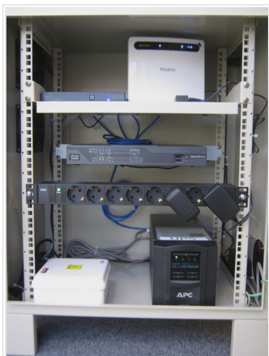
Fig. 2 - Interior de rack AD Rural
